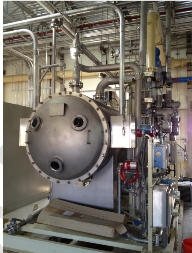
Figure 5-3 Ozone Generator (1,200 ppd)
