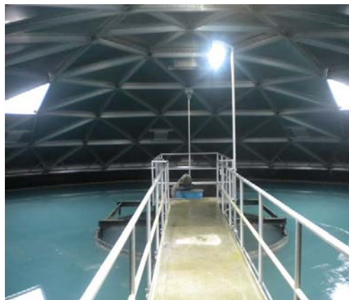
Figure 5-8: Dewatering Facility Thickener
