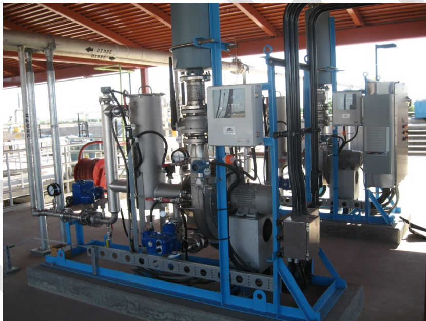
Figure 5-4 Catalytic Ozone Destruct Unit
