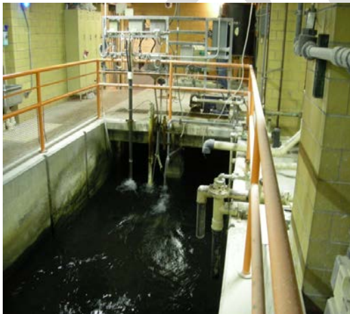
Figure 5-1: Rapid Mix Channel
