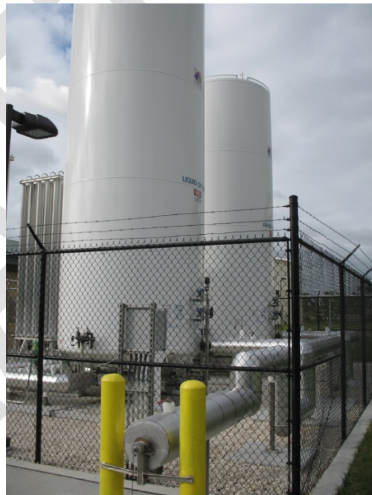
Figure 5-1 Vertical LOX Storage Tanks
